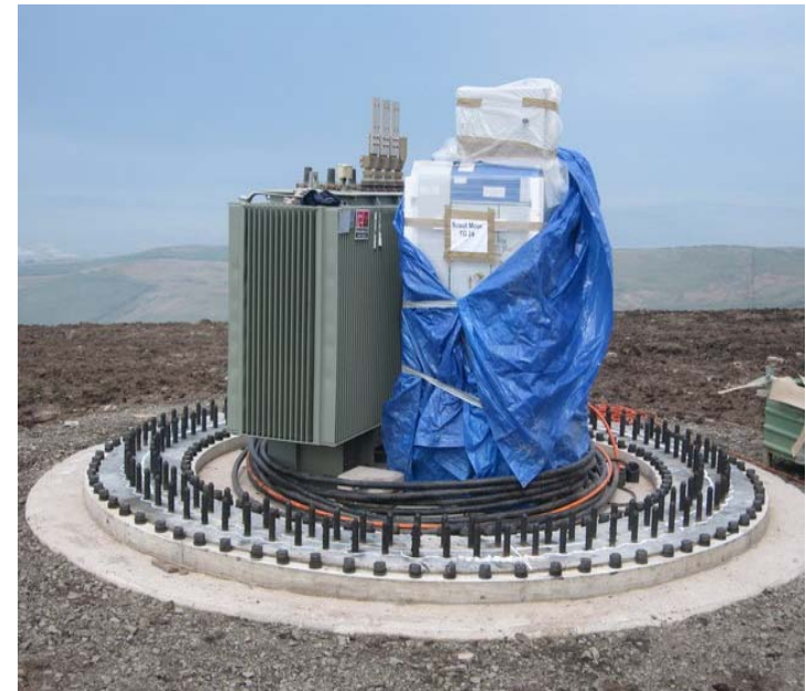
Turbine base and transformer (Photo: P. Anderson)
