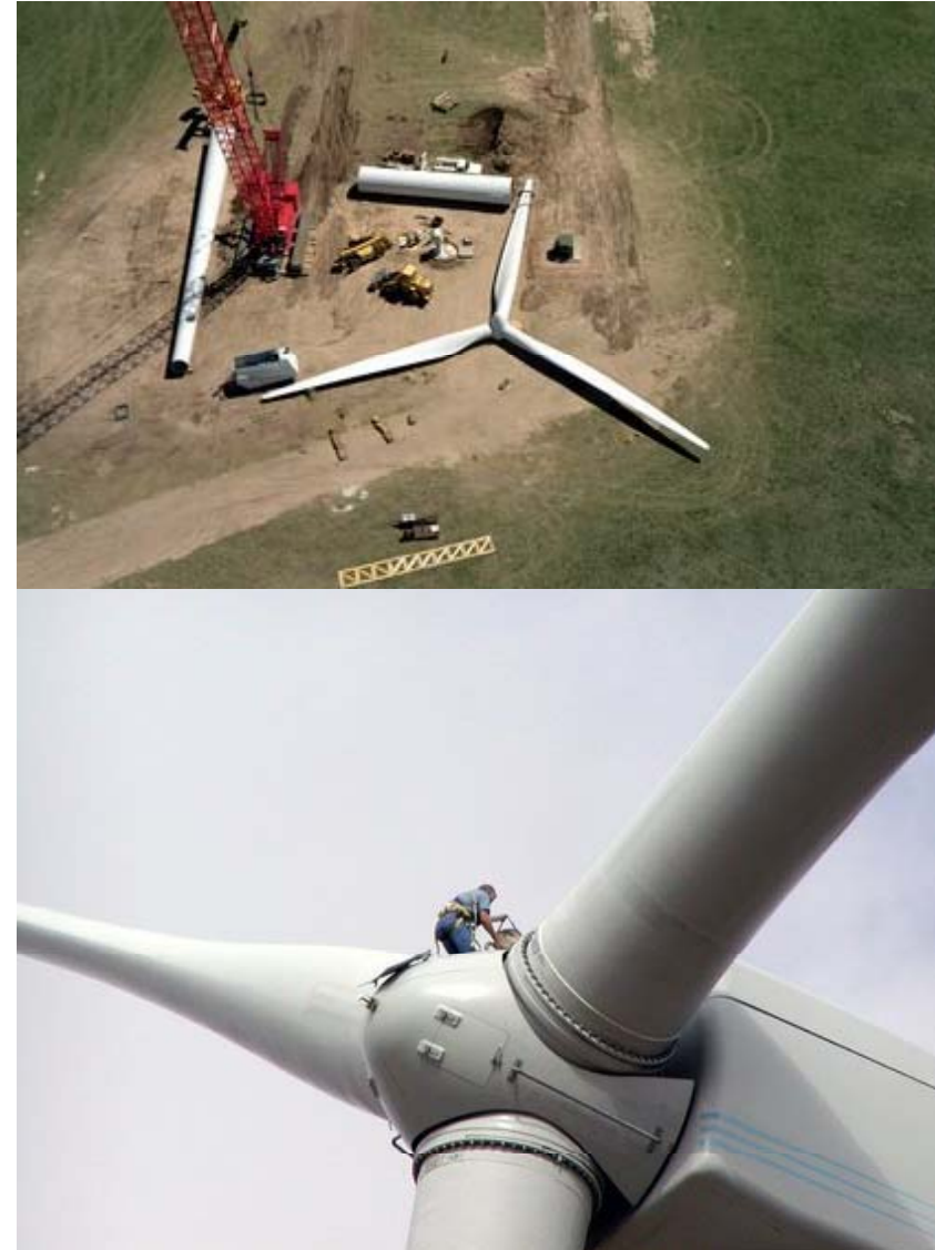
Researcher entering the hub of a GE Wind (formerly Enron Wind) 1.5 MW wind turbine (DOE/NREL, Sandia National Laboratories)
