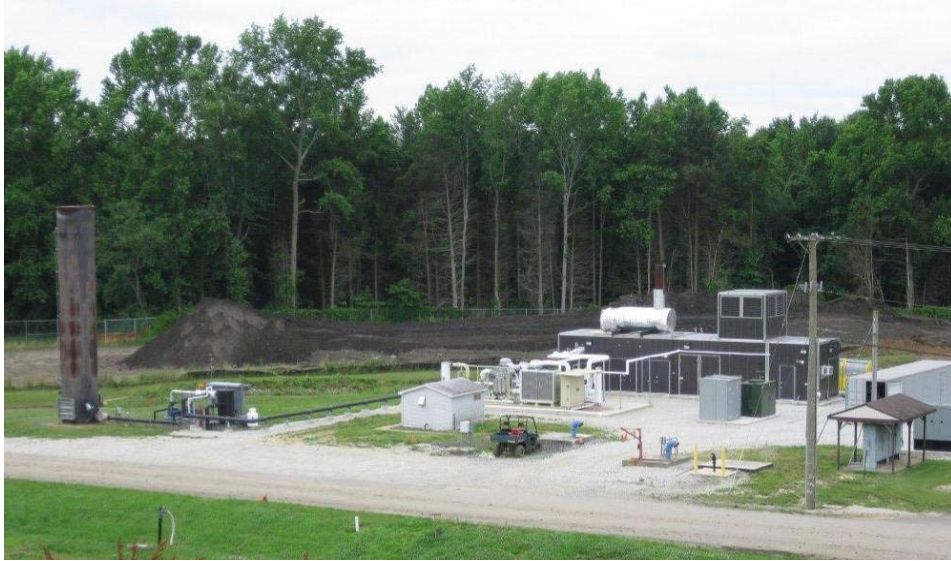
Figure 3-3. 1.6 MW LFG Reciprocating Engine Housing (DCO energy).
