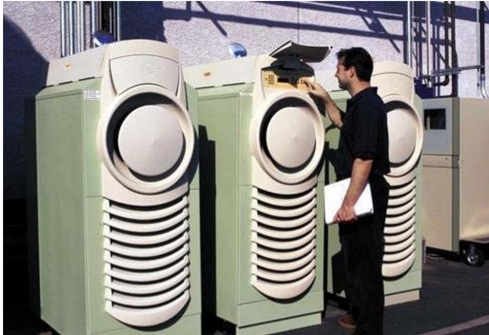
Figure 3-4. Capstone Microturbines (30 kW).
