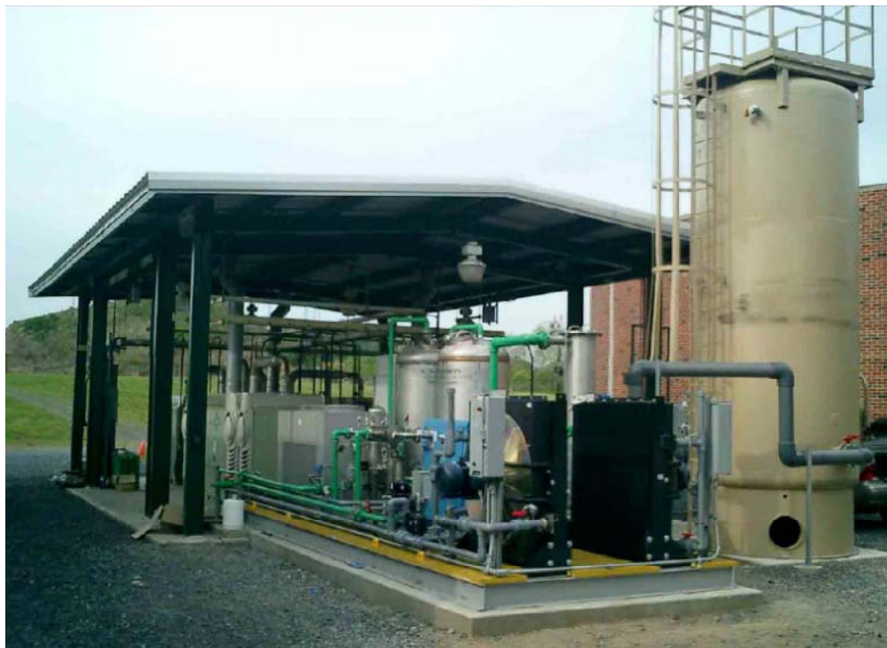
Figure 3-5. Capstone Microturbines and Gas Treatment Skid Outdoor Installation.
