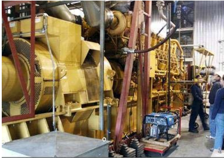
Figure 3-2. Reciprocating Internal Combustion Engine Utilizing LFG.
