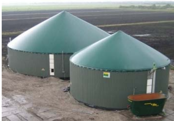
Figure 3-9. Complete Mix Reactors - 526 kW plant (courtesy Biogas Nord).
